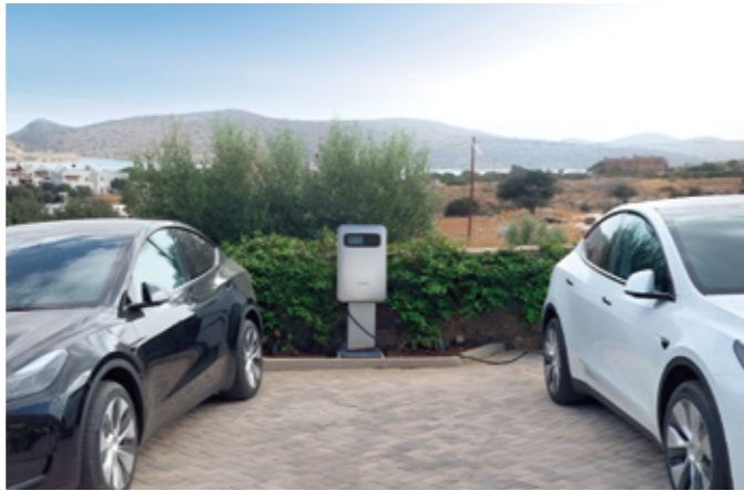
Resort EV charging station in Crete, Greece
