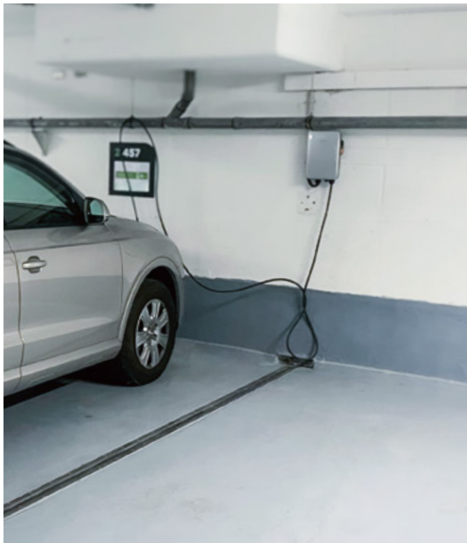
Office area EV charging station in Munich, Germany
