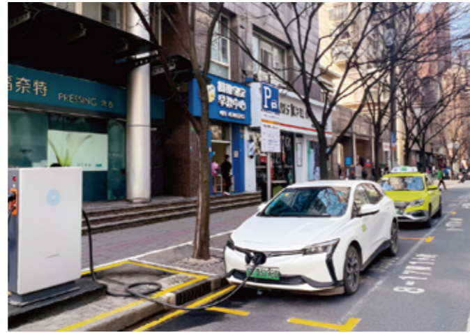
The first on-street parking EV charging station in Shanghai, China
