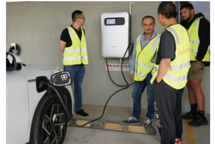
Warehouse EV charging station in Sydney, Australia
