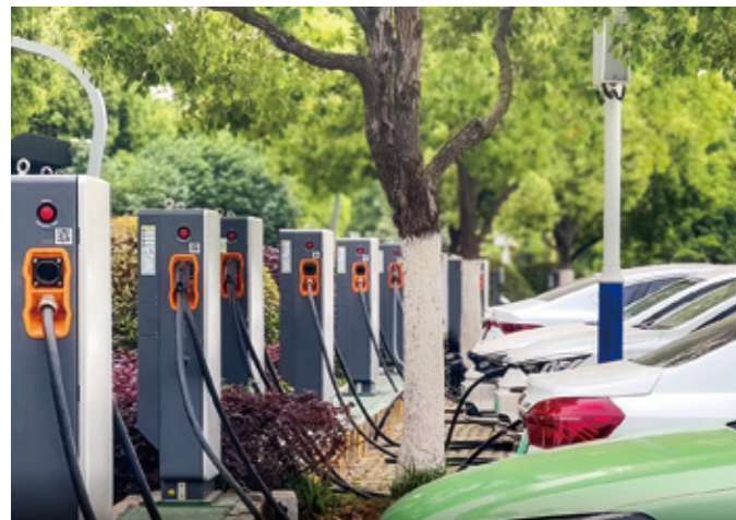
Tangxihe Park fast EV charging station in Anhui province, China
