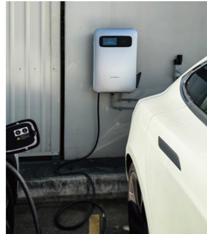
Public EV charging station in Australia
