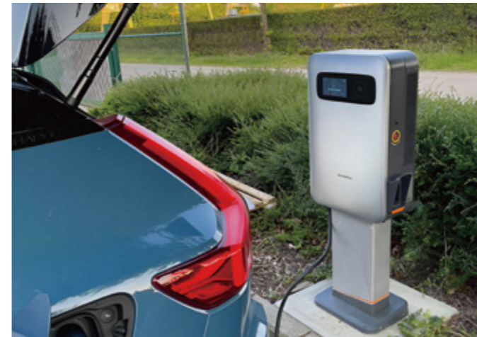
Workplace EV charging station in Herentals, Belgium
