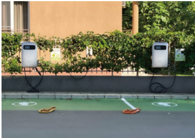
Sunny beach EV charging station in Bulgaria
