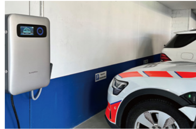
Police EV charging station in Muri, Switzerland
