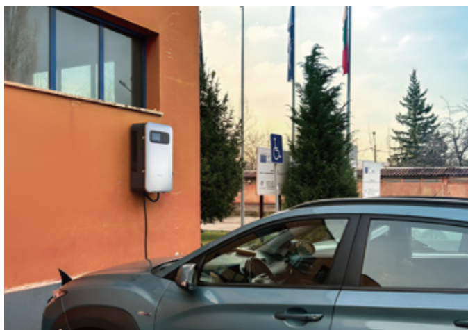
Factory EV charging station in Pernik, Bulgaria
