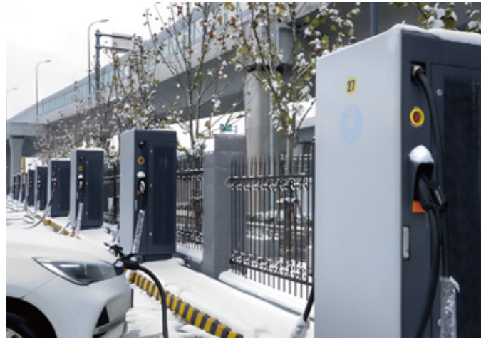
Leshui public fast EV charging station in Anhui province, China
