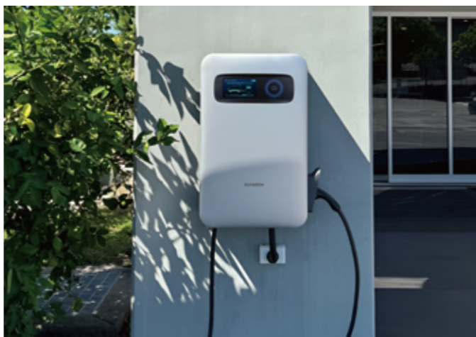
Office EV charging station in Australia
