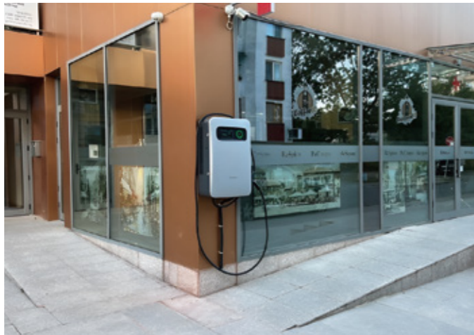
Medical center EV charging station in Razgrad, Bulgaria
